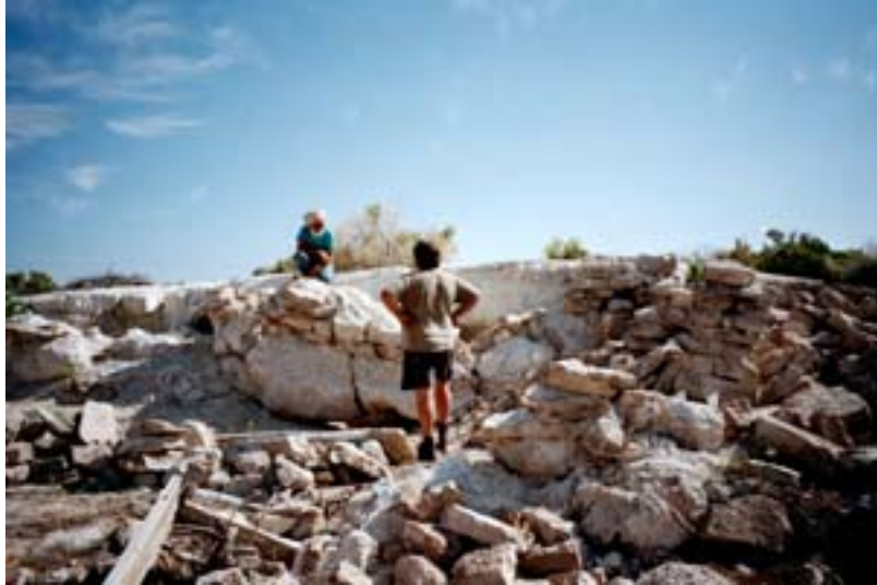
First day on the project, assessing the rear wall where the mound has collapsed (FWS 23691-3).
