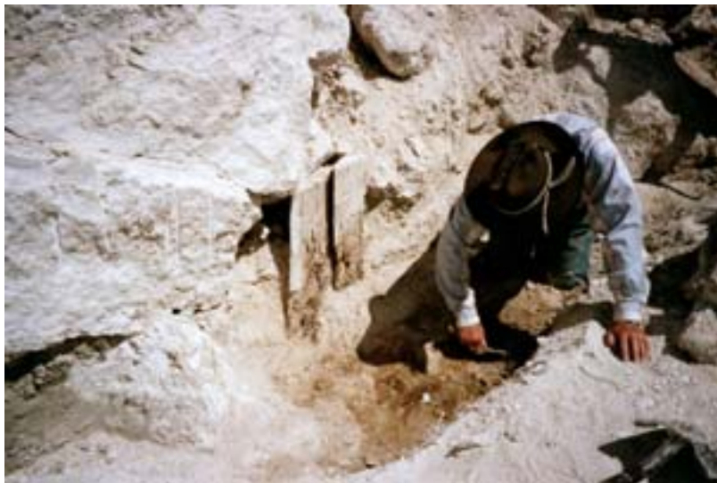
Erich Obermayr excavating new foundation trench along rear wall after spring mound boulders were removed (FWS).
